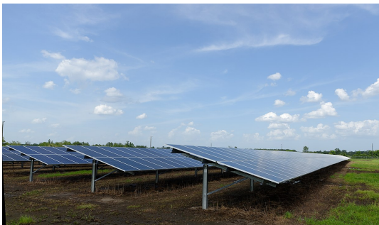
Figure: Solar panels
